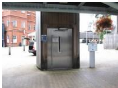
Access lift to high level walkway
